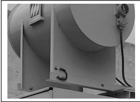
Figure 81: Union conservator tank with main tank
