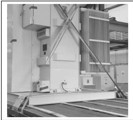
Figure 26: Wooden boards between the metal base of the transformer and the metal floor of the truck
