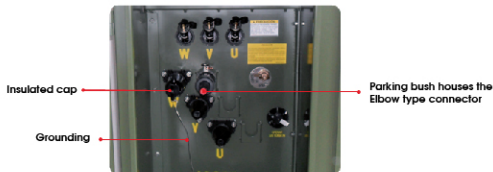
Photograph 2. Pad with Insulated cap and parking bush
